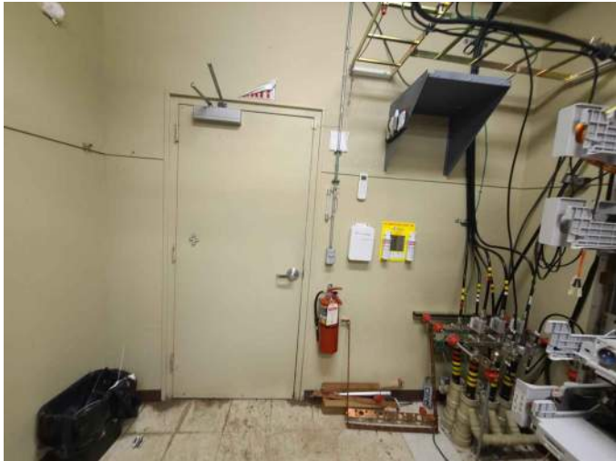
D EX. SHELTER ACCESS SCALE: NONE
