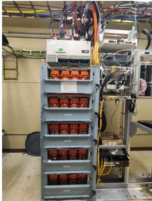
E EX. BATTERY RACK SCALE: NONE
